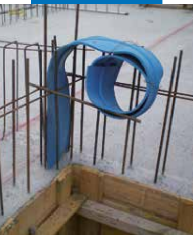
Structural joints in a wall with a PVC profile embedded in the foundation pad after casting
