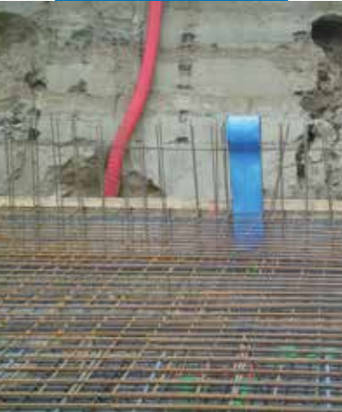
Structural joints in a wall with a PVC profile embedded in the foundation pad before casting
