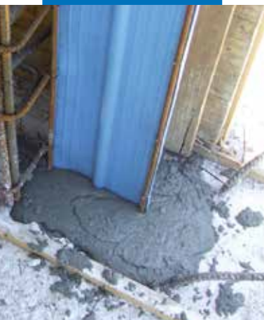
Idrostop PVC BI embedded in the foundation pad with Mapegrout Hi-Flow before demolishing part of it
